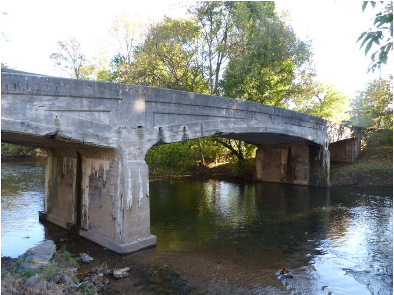
Lancaster County, Pennsylvania is home to two bridges that are the only known surviving bridges to even come close to the design of the Adamsville Bridge. This is the Farmersville Road Bridge, and it is slated for demolition and replacement. It was built in 1917.
