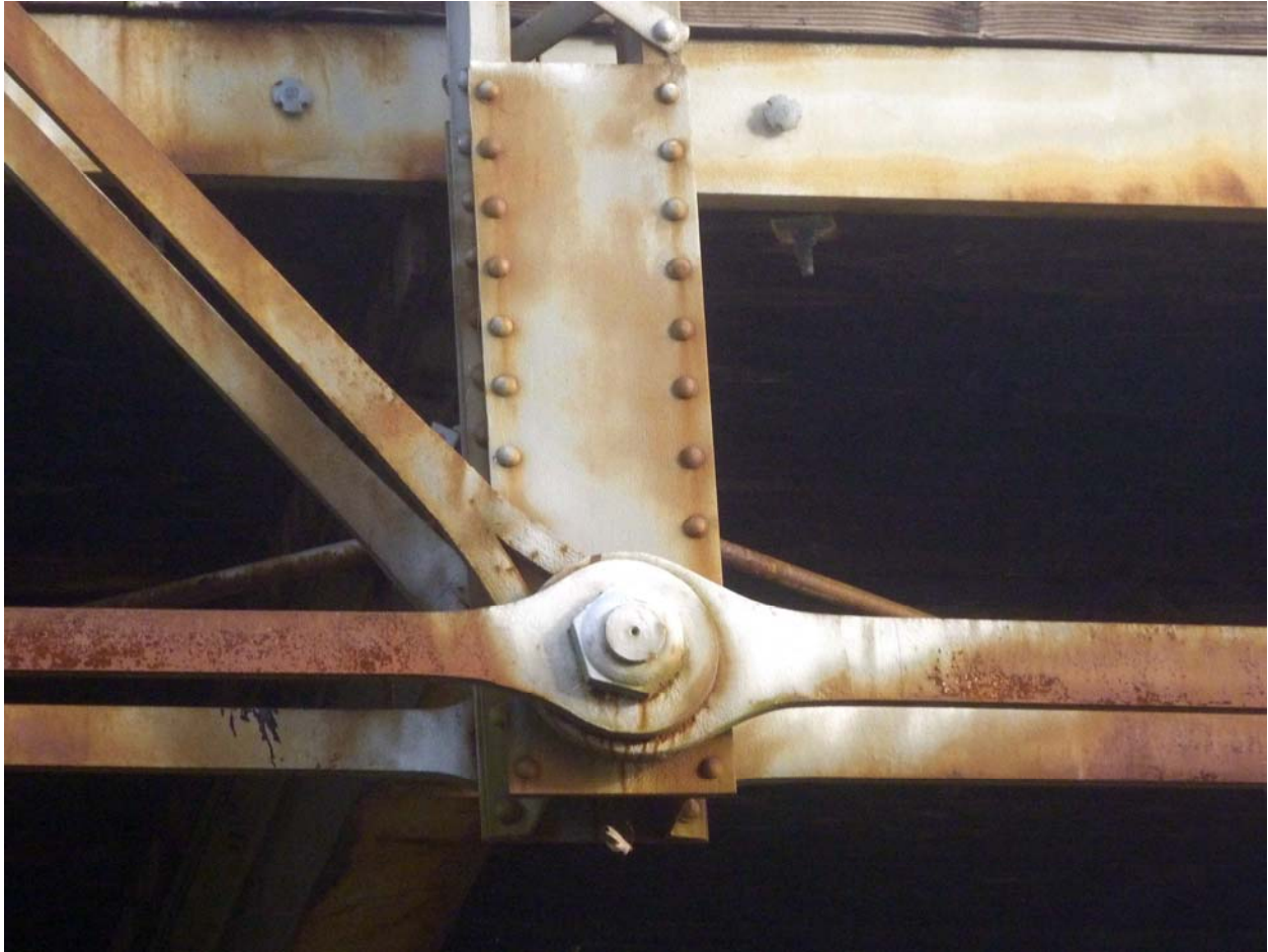
6- Bottom chord connection on bridge. Here, the bottom chord is composed of up-set eyebars, while the diagonal member is composed of loop-forged eyebars.
