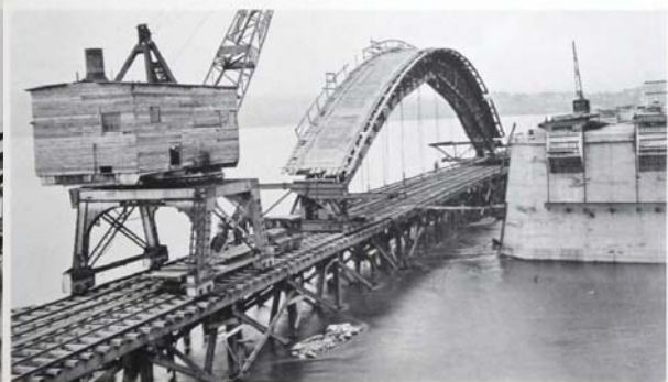
Columbia-Wrightsville Bridge over Susquehanna River. Blaw-Knox Steel Centers ready to be rolled in position between piers.
