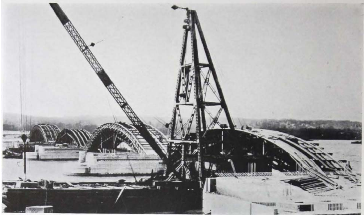
Arlington Memorial Bridge, Washington, D. C. Hunkin-Conkey Construction Company, contractor. Eight spans, barrel type arches. Minimum spans 166', Maximum spans 180', width of arch 94'. Blaw-Knox steel centering furnished for four spans one-fourth width of arch.
