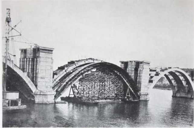
Key Bridge, Georgetown Washington, D. C. U. S. Engineering Corps. Blaw-Knox steel covering for 200' clear span being lowered with floating equipment using tide or crane and lower centering.
