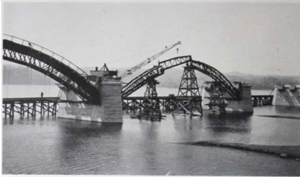
Columbia-Wrightsville Bridge over Susquehanna River, Wiley-Mason Company, contractor, showing method of erecting twin trusses on 185' spans.
