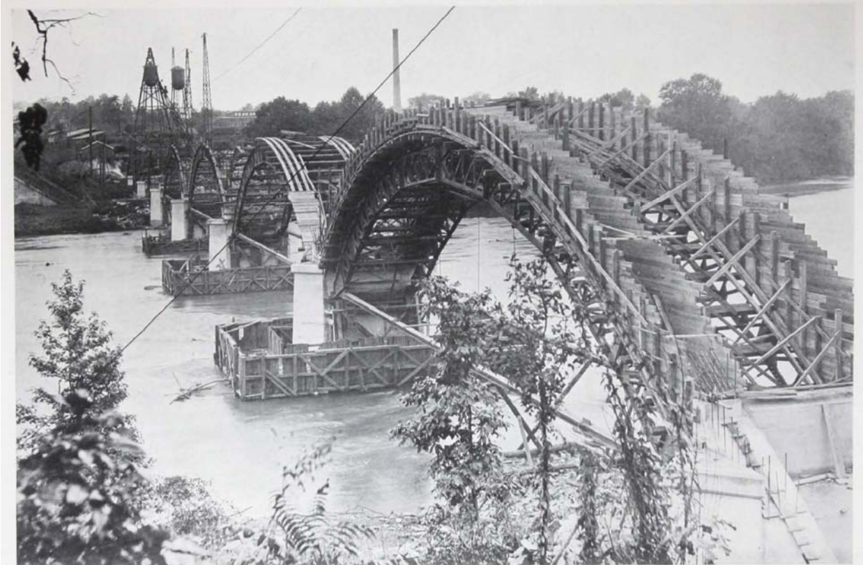
Yadkin River Bridge, Yadkin, N. C. Hardaway Contracting Company, Inc., contractor. Blaw-Knox centering furnished for full width of bridge. Seven 150' spans. Rib type arches.
