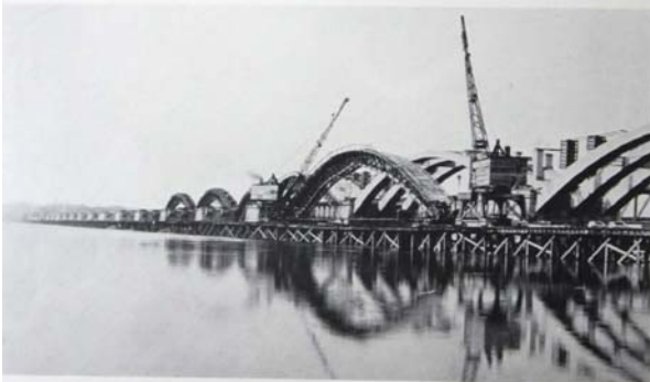
Columbia-Wrightsville Bridge over Susquehanna River. Blaw-Knox Steel Centers are being rolled laterally onto construction trestle.
