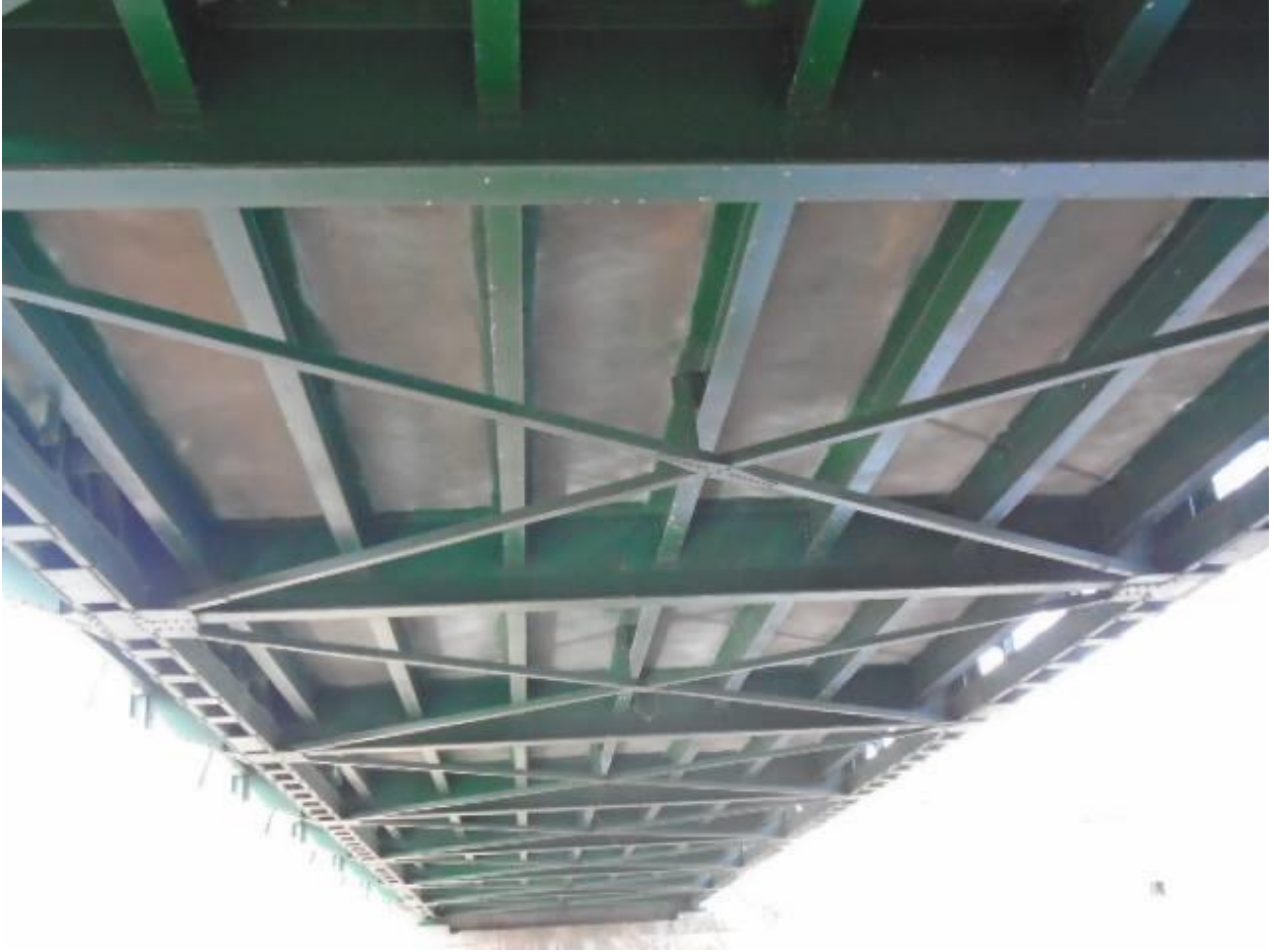
View under bridge showing deck stringers, floor beams, and lower lateral bracing.
