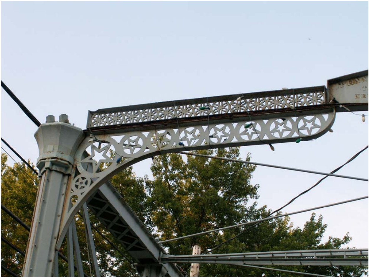
Ornamental portal bracing detail for the Whipple truss. The portal bracing is cast iron.
