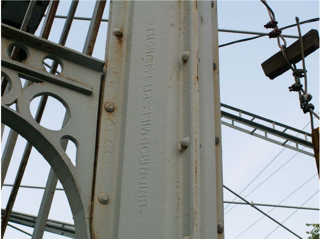
A Keystone Column on the bridge's Whipple truss with a brand indicating that it was rolled by the Union Iron Mills of Pittsburgh
