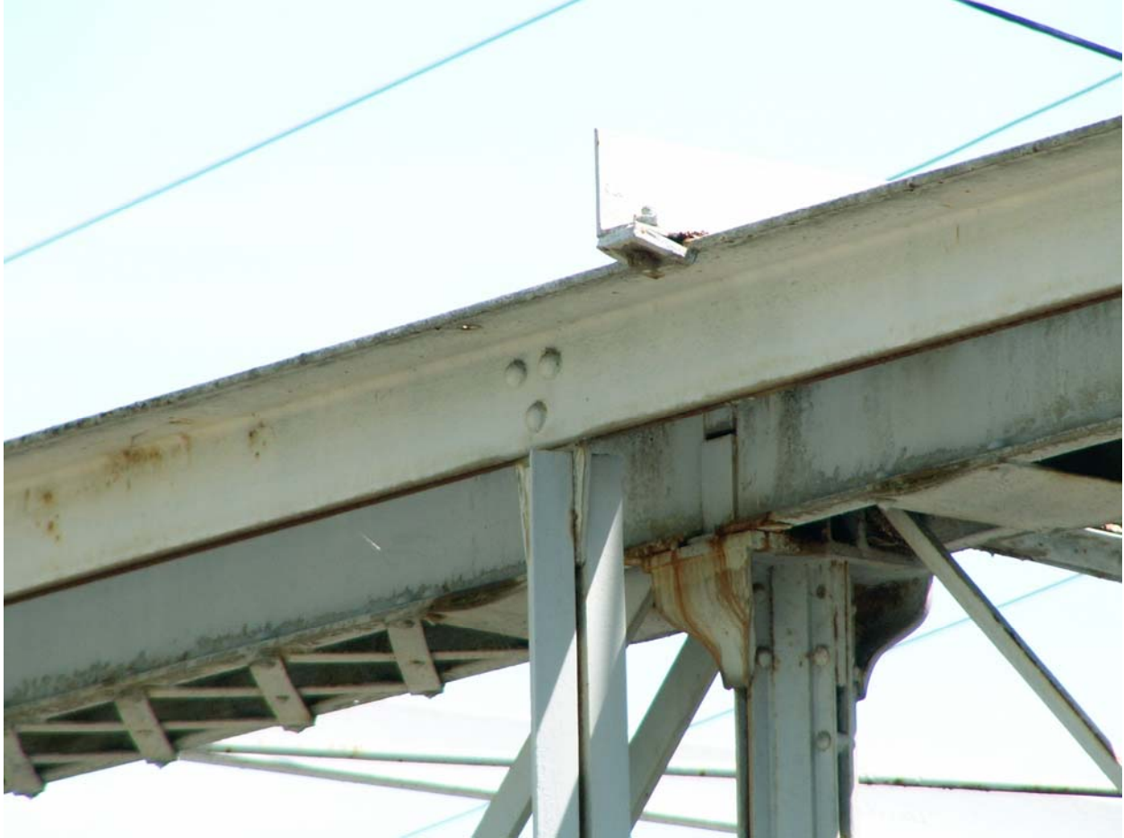
Top chord connections. The Baltimore truss connection is shown to the left and the Whipple top chord connection is shown to the right.
