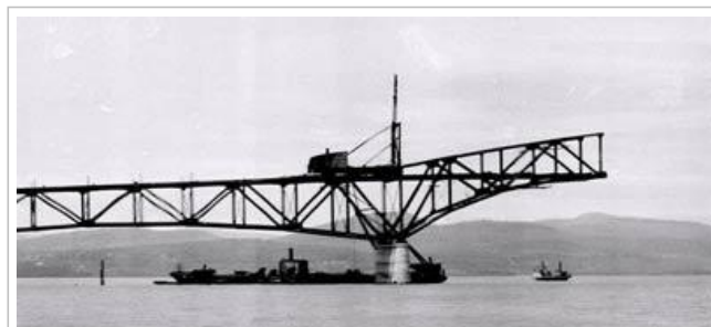
Innovative construction methods allowed the erection of cantilevered steel chords without the need for temporary supports. Photo courtesy of Vermont State Archives.
